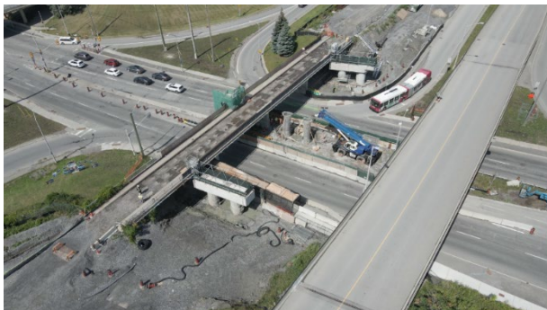
Pictured above: Support column work has started at the Hunt Club rail over road bridge.
